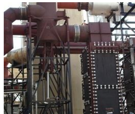
Waste heat Recovery unit (HRU)
