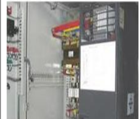
VFD for paint shop blowers
