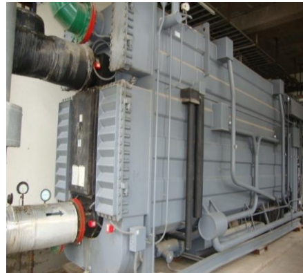
VAM for Plant Air Conditioning
